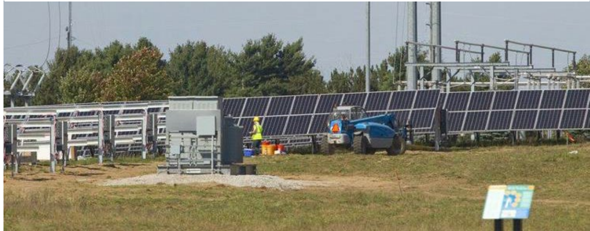
Solar Array owned by Heritage Sustainable Energy, Traverse City, MI
